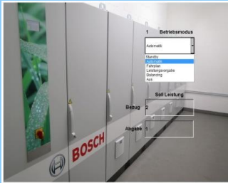
135 kWh Kelsterbach, DE, Community storage
