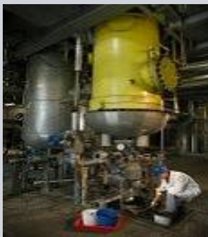
Siemens Fuel Gasifier
