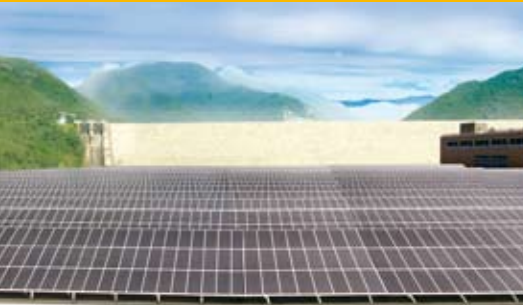
Solar plant in Korea
