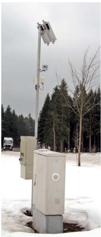
Black ice early warning system with wireless M2M communication.
